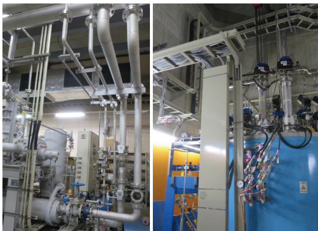
Fig. 1. New cooling water piping for the compressor and refrigerator.
